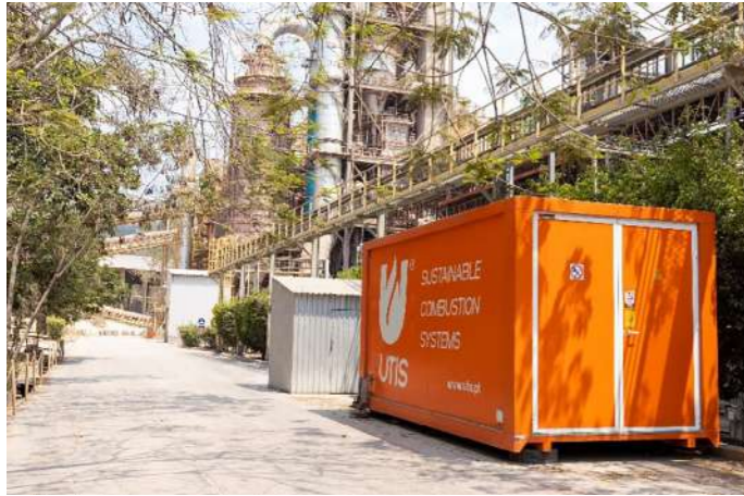
Hydrogen injection in Piedras Azules Plant, Honduras
